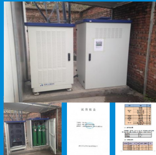
Backup power source for communication China Mobile Base Station Operation in Dazhou, Sichuan
