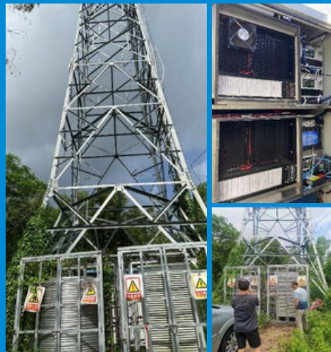
Backup power source for telecom services Demonstration unit in Doushan Base Station in Jiangmen, Guangdong
